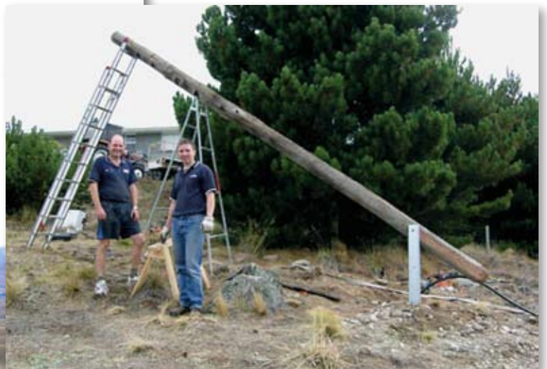
INSTALLING THE NEW TEKAPO TOURISM WEBCAM. ABOVE: GREG KNOWLES AND TIM RAYWORD LEFT: UP THE LADDER GREG KNOWLES - BELOW TIM RAYWARD
